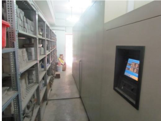
Centralised AC for controlling the temperature and humidity of the labs
